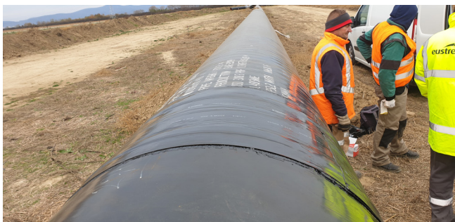
Figure 2. Asset operator, contractor and coating supplier evaluation after coating the field joint.
